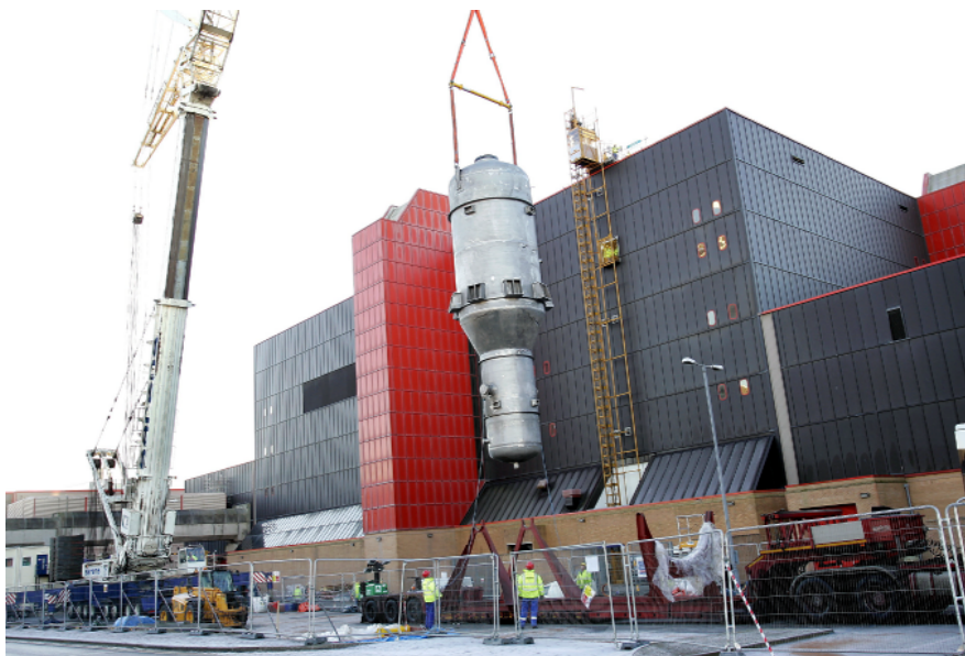
One of the four vessels being lifted into Thorp earlier this year
