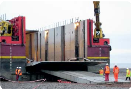
Door almost down
